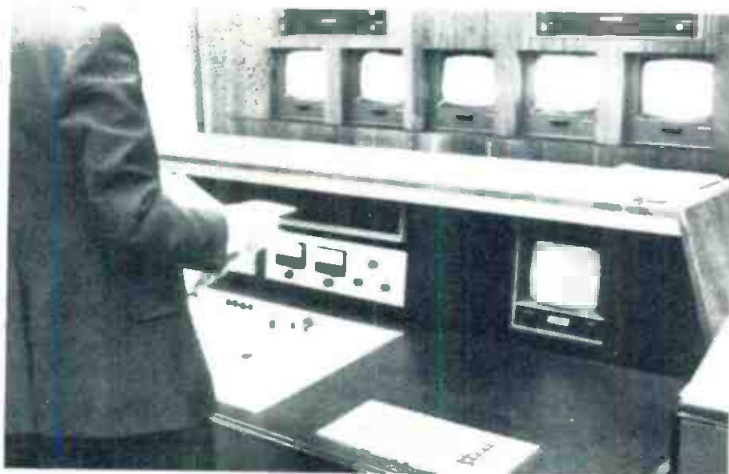
Grass Valley's TV switching automation system.
